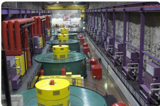
Generator room inside the mountain (TVA photo).
